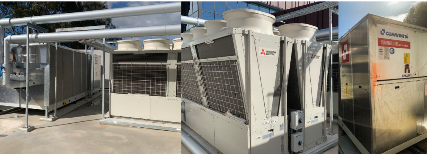
ERACS2 System & E-Series units providing hot water supply.
