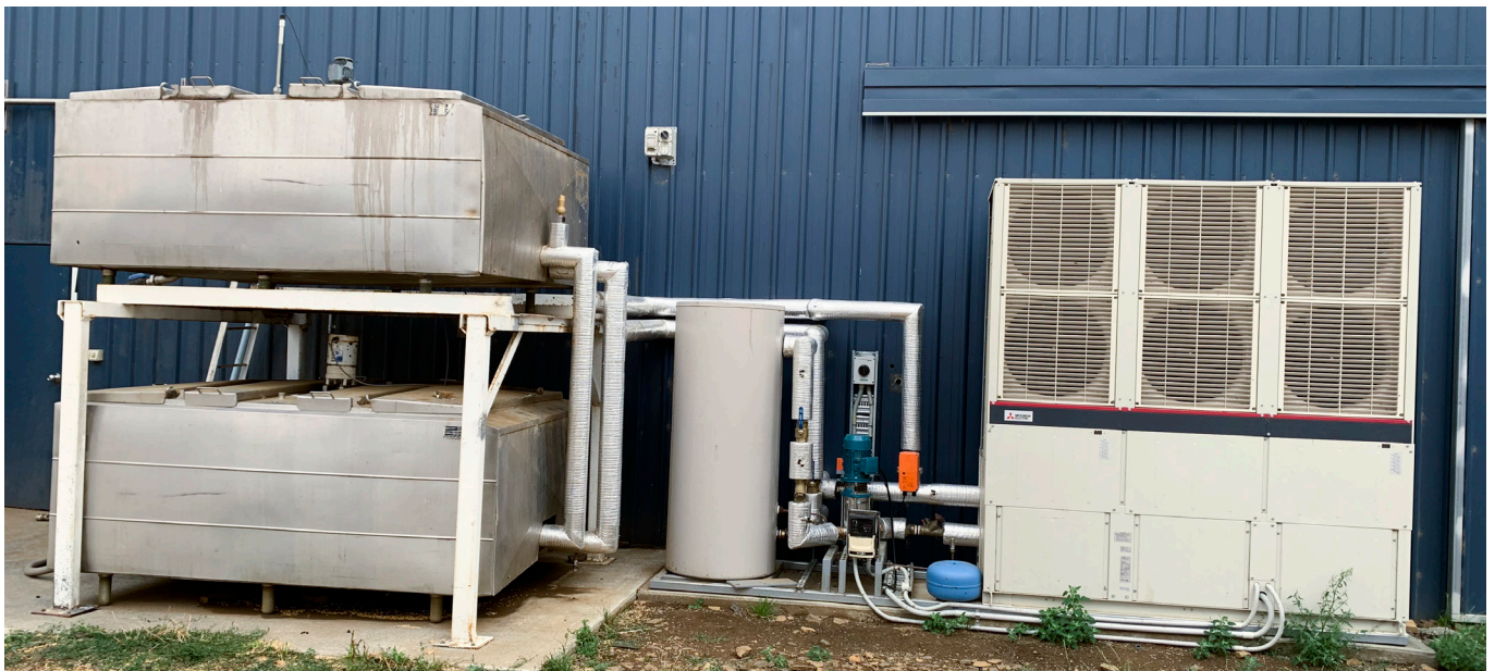
e-series chiller, buffer tank and calf milk vat 1 & 2
