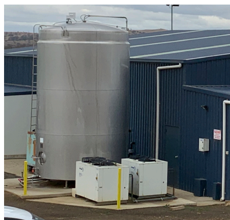
Bulk tank and DX chiller
