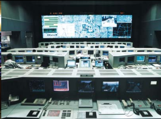
Police command & control room
