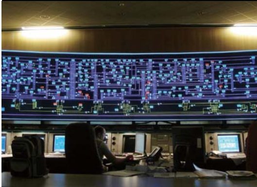
Electric utility control room
