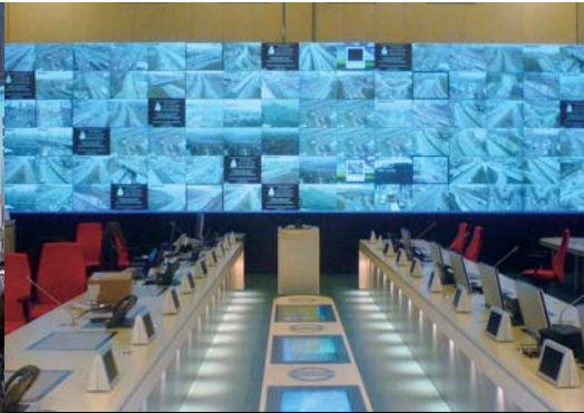
Traffic control room
