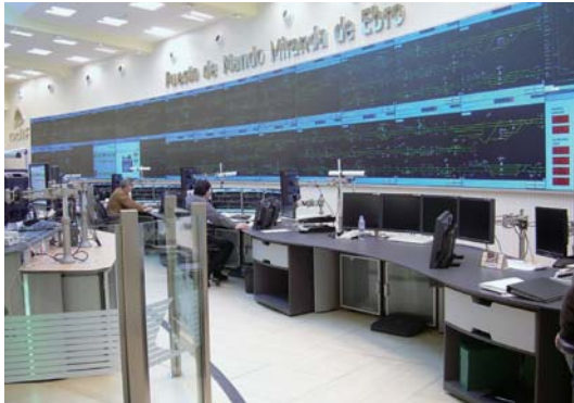
Railway control room
